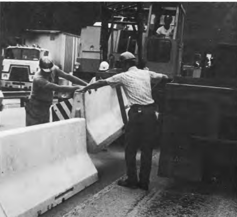
The ESI safety barrier being installed on a section of the Pennsylvania Turnpike.
