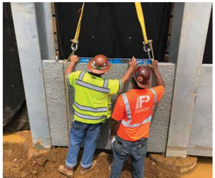
Smith-Midland is manufacturing more than 1 million square feet of sound walls and retaining walls for the Transform 66 project near Washington, D.C.
