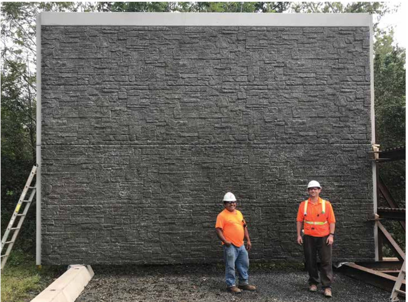
Installation and manufacturing of the panels continues, and the project is scheduled to be complete in 2022.
