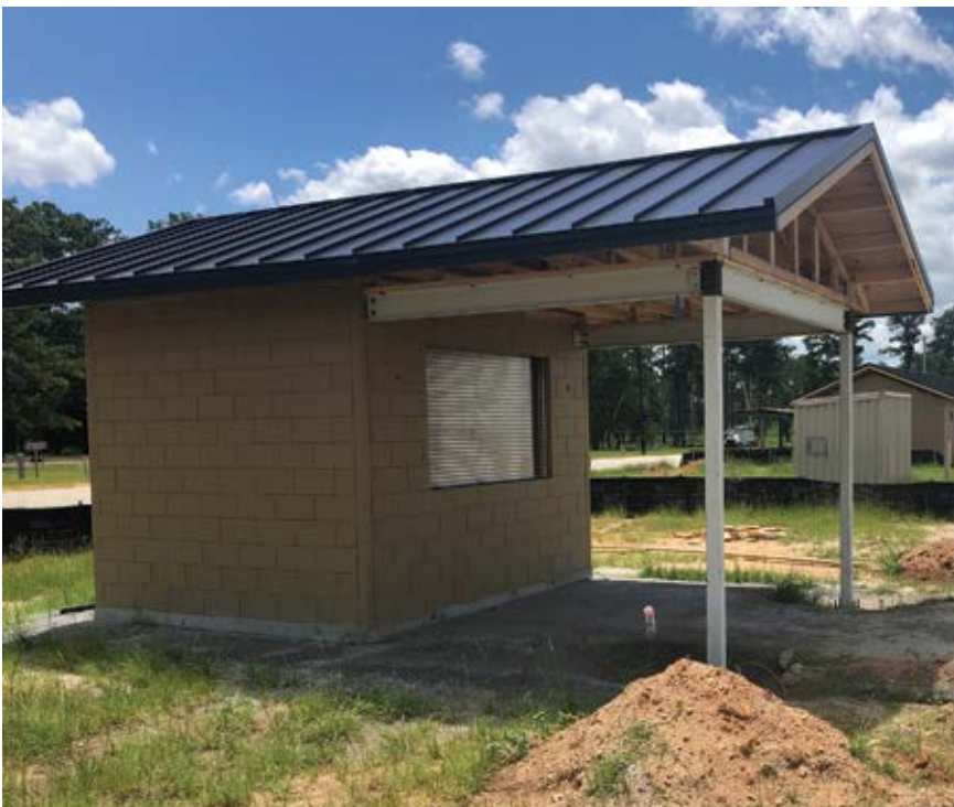
The precast facades were made to look like hand-laid masonry to match the existing architecture. By using precast, the project was completed in just a few months.
