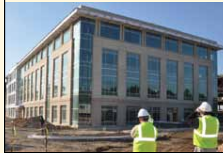
NBP 430 - Annapolis Junction, MD architectural precast 18,931 sf 90% complete Client: Hitt Contracting Corp.
