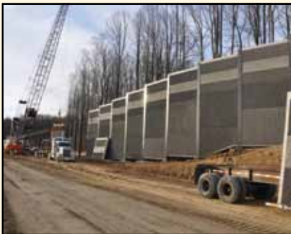
Intercounty Connector: Contract B (ICC-B) Montgomery County, MD: Soundwall 762,186 sf 90% complete Client: Kiewit Construction
