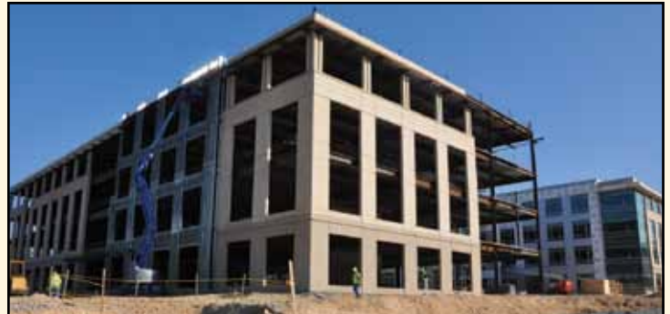
National Business Park (NBP) 410 - Annapolis Junction, MD: architectural precast - 19,000 sf 100% complete; Client: Hitt Contracting Corp.
