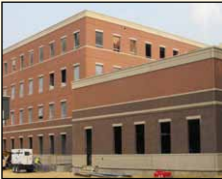
U.S. Army Legal Services Agency & Army Audit Agency (USALSA) Ft. Belvoir, VA: Slenderwall 33,400 sf 100% complete Client: Suffolk Construction
