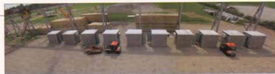
These Easi-Set precast concrete buildings, manufactured by Lonestar Prestress Mfg., Inc., were delivered in July as part of a City of Houston public works project. The buildings, engineered to withstand 140mph winds, house communications and Supervisory Control and Data Acquisition (SCADA) equipment for the Houston groundwater infrastructure upgrade project.
