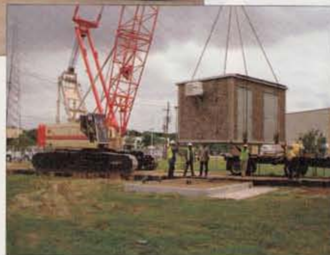
Lonestar Prestress' 10x14x8 foot Easi-Set building being offloaded at a Houston groundwater facility onto a prepared foundation consisting of precast retaining walls backfilled with pea gravel.
