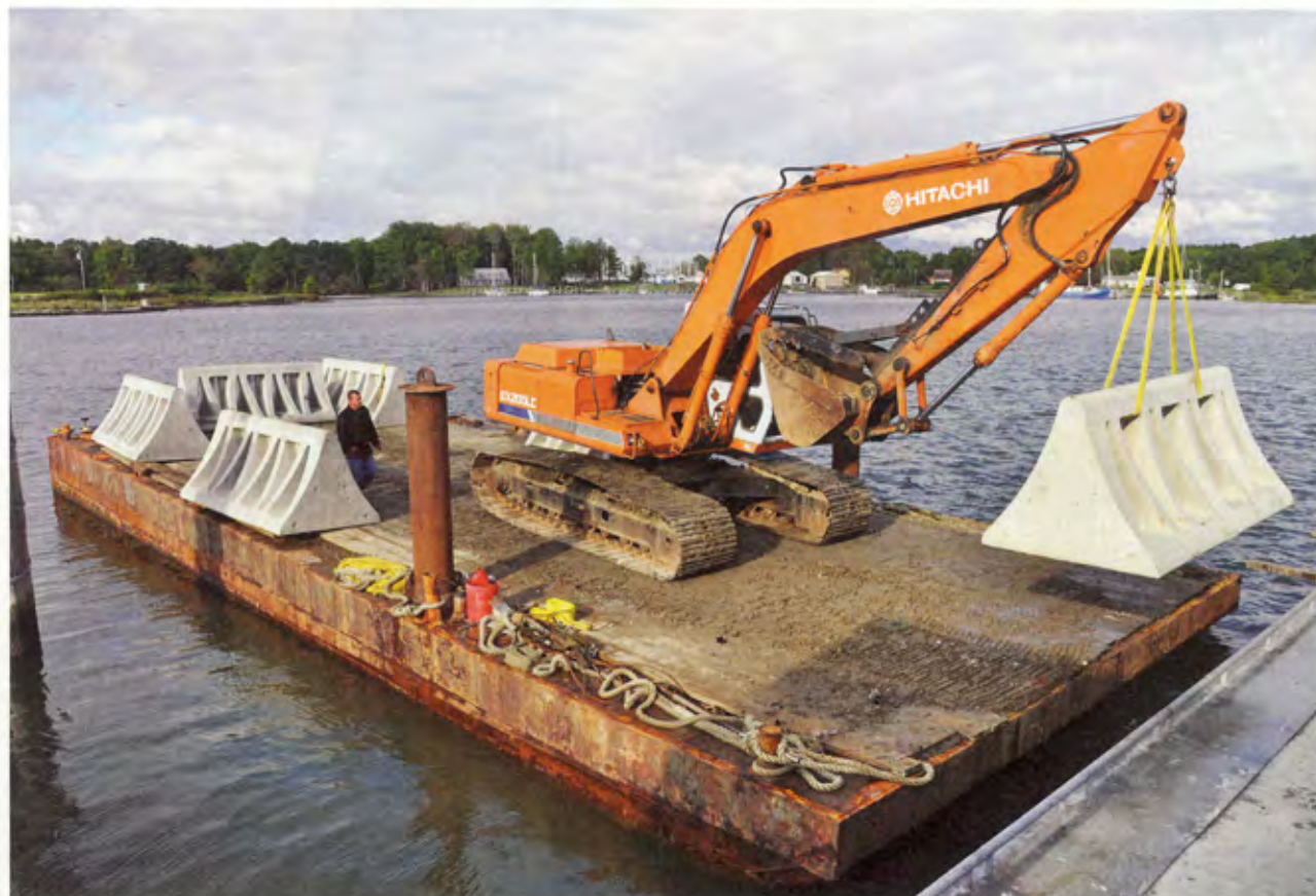
A Virginia couple has Beach Prisms installed in their home on Chesapeake Bay to reduce beach erosion. Courtesy of Smith-Midland Corp.
